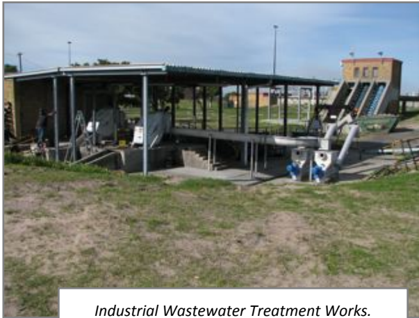
Industrial Wastewater Treatment Works.
