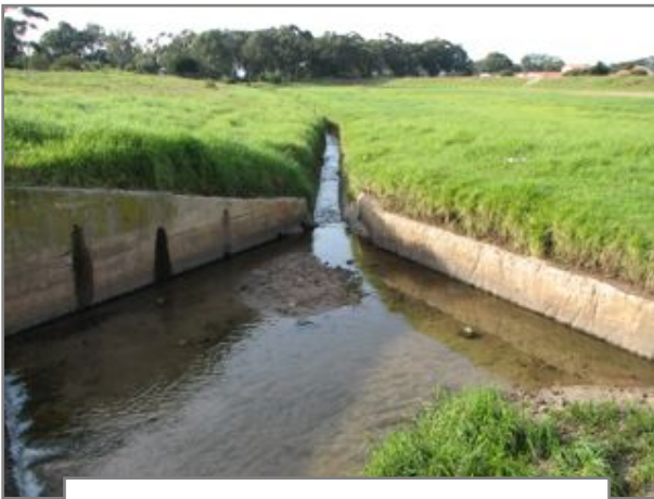
Basin 3: Storm water inlet.
