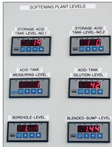
Water softening plant: water level monitoring.
