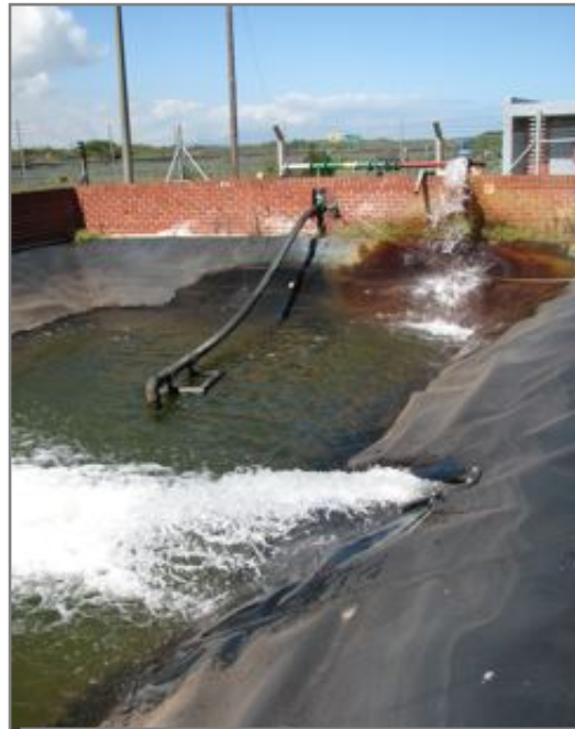
Waste acid pond: backwash brine from regeneration process (right); dilution water from borehole (back right); disposal pipeline suction (black pipe).
